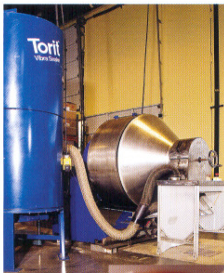
A point-of-source vacuum reduces dust associated with discharge.
